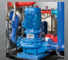
Jacket Water Pump
