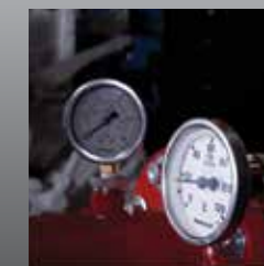
Temperature and Pressure Gauges
